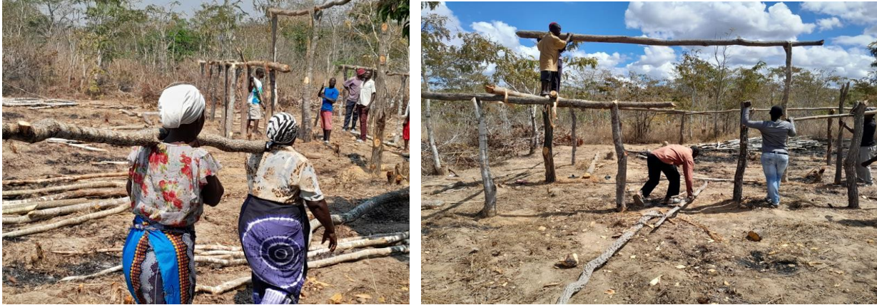
Image 7: Engagement of women and men in the construction of an annex classroom in the Chinhamudidi neighbourhood, Guindingue community
